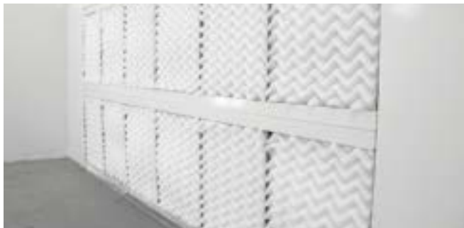
Exhaust filters on wall
